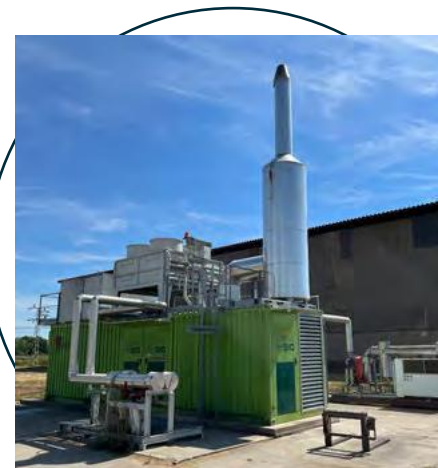
Biogas generator, Statek Kravaře, Czech Republic
