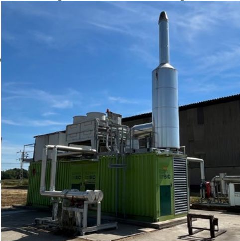
Biogas generator at Kravaře Farm, Czech Republic
