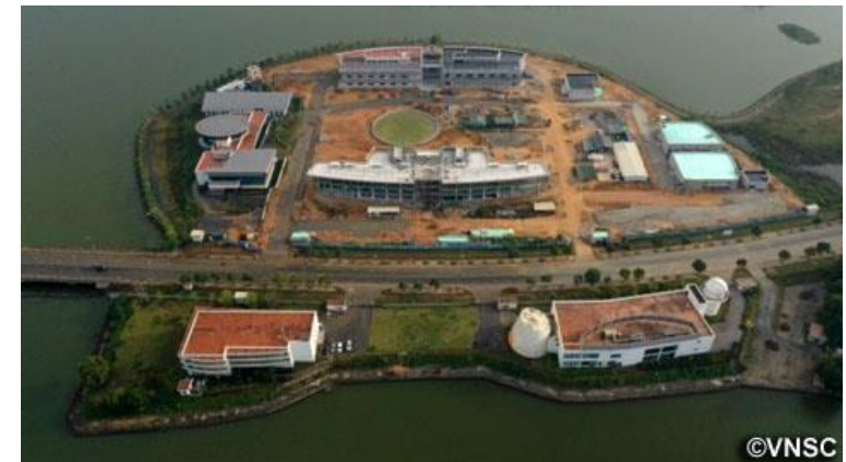
Vietnam National Space Center construction site in Hoa Lac Hi-Tech Park (Photo by Vietnam National Space Center)
