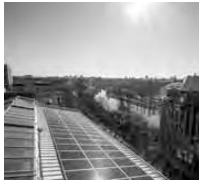
GSG Solar PV, Berlin, Germany
