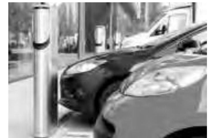
Charging station at Eurocentrum, Warsaw, Poland
