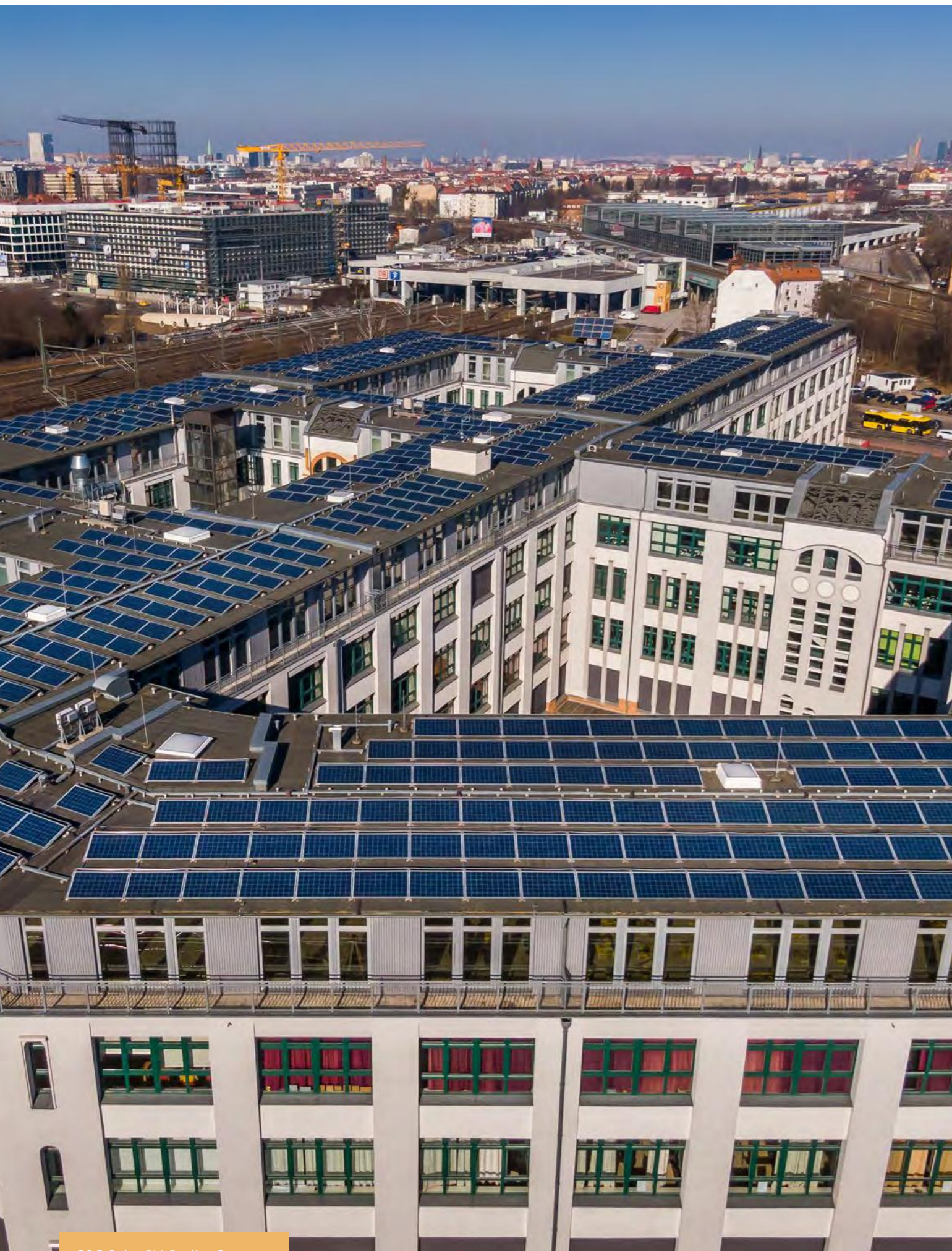
GSG Solar PV, Berlin, Germany
